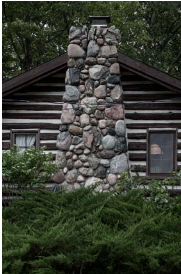
Rock collecting. Kay gathered rocks from near and far to be included in the restoration of the chimney.
