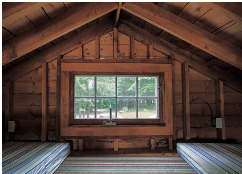
Flop on top. The unfinished loft above the living room provides ample (albeit spartan) space for overnight guests, with a view over the living room below.
