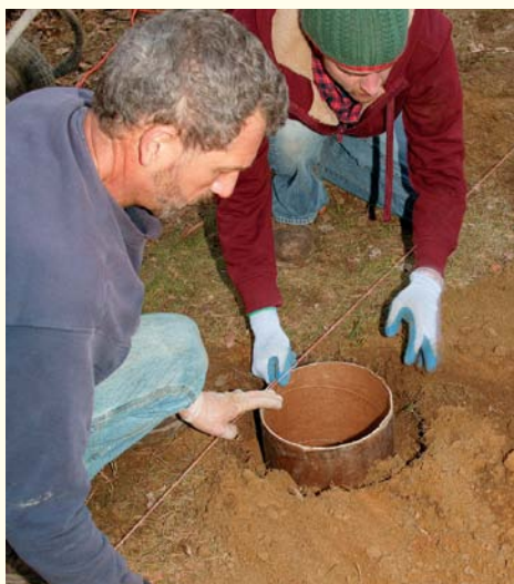
The footings must be located directly below the beam. After placing the bags and tubes, pour enough concrete to fill the bags up to the cardboard tubes. Then reset the string, align the tubes to the center of the beam, and backfill around the tubes.
