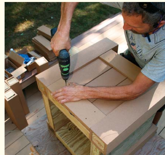
Box the panel. Apply horizontal trim boards across the top and bottom of each panel. The horizontals and the post sides are in the same plane and complete the frame.
