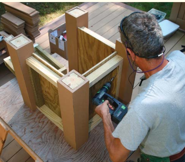
A solid framework. As a smaller version of the half-wall construction, the first stage of the planters is built with panels made from 2x2s and plywood that are screwed to corner posts. After assembling the box, add a second layer of plywood to the outside of the frame.
