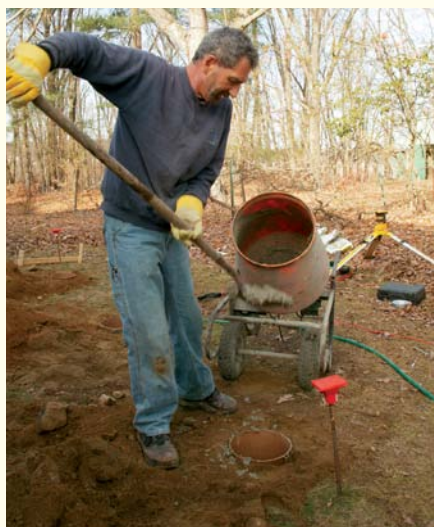
Site-mixed concrete. Mix concrete in a wheelbarrow-style mixer, then shovel it directly into each form. When all are filled, reset the string, and place the J-bolts in the wet mix directly below the string.
