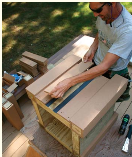
First layer of trim. Clad the exterior of each panel with trim boards backed with strips of joist tape at gap locations. Fasten the boards with trim-head screws.
