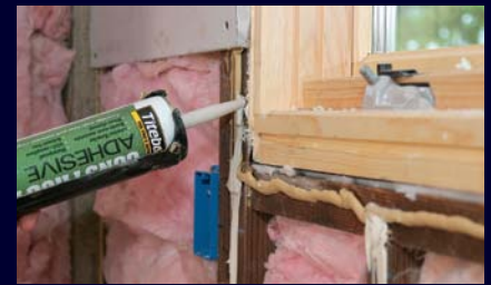
Drywall air barrier. Finished wallboard is mostly free of holes and can be made into an excellent air barrier by sealing around fixture boxes and along untaped seams. Caulk or adhesive on the framing prevents air movement.
