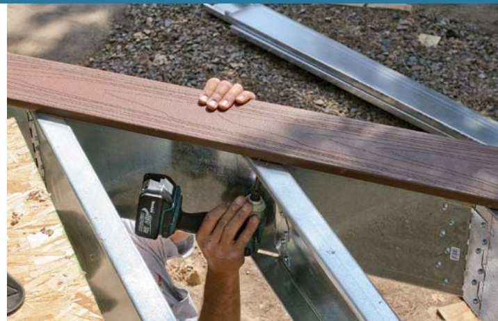
Fasten from below. Short galvanized screws through joist flanges from below hold the edge boards.
