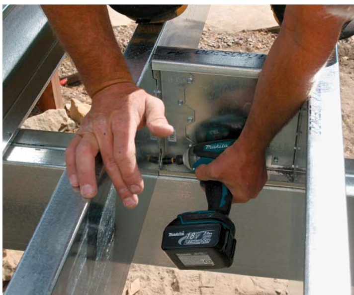
Block between the joists. Self-tapping screws fasten framing angles to blocking and to the joists. Two additional screws secure the blocking to the beam.
