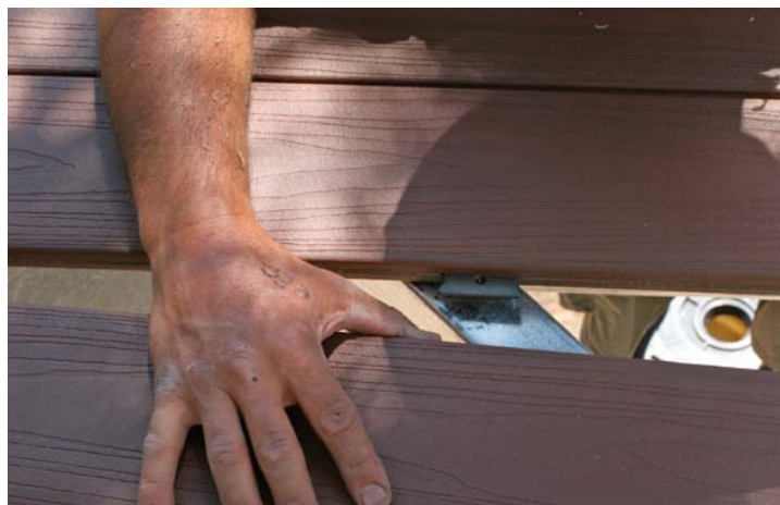
Hidden fasteners work well with steel framing. The key is to use a biscuit-type fastener that relies on a vertically driven galvanized screw, not an angled screw, which won't engage in steel framing.
