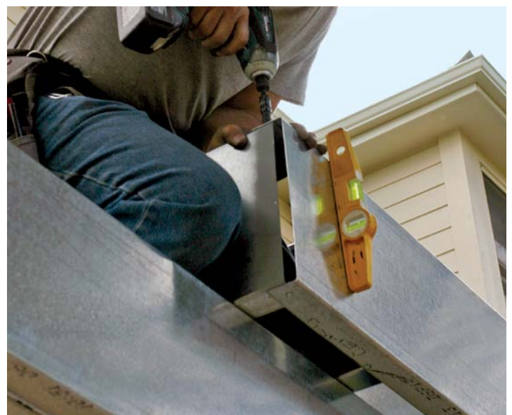
Screw rim to joists. Sight along the rim as you screw it to the joists to keep the edge of the deck straight.
