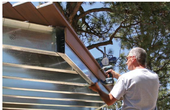
Cover the steel. Fascia material—in this case, a pair of deck boards—hides the shiny rim joist from view.
