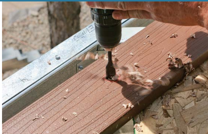
Counterbore for protruding screws. To keep the decking from rocking on the screws holding the rim to the joists, drill shallow holes in the bottom of the decking.
