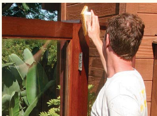
Use a small pad for small spaces. A disposable, handheld painting pad is good for applying finish to areas too small to spray and too big to brush.
