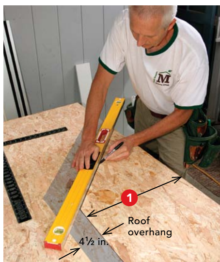
Add the overhang. Draw the window shape onto the OSB template, and add the 4 1/2-in. roof overhang to the front and sides of the template.
