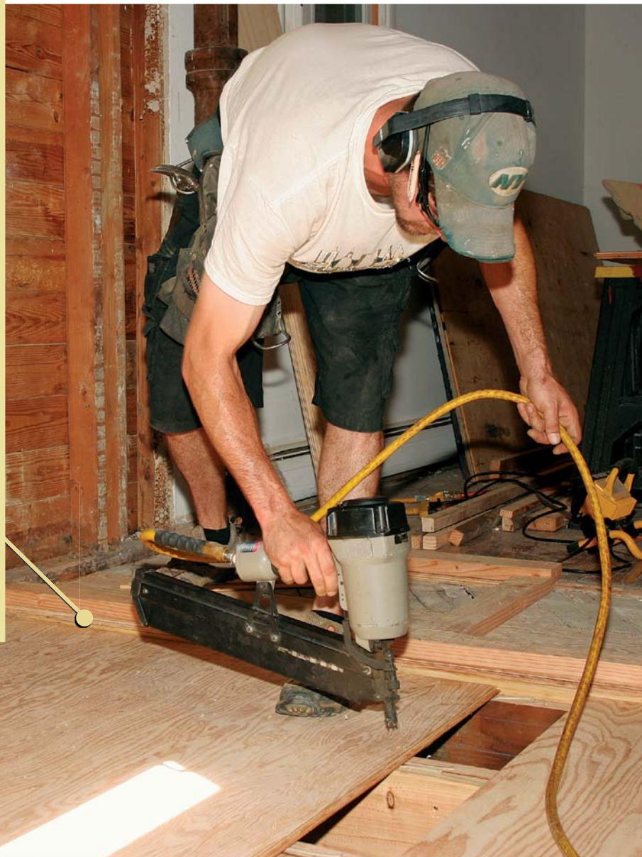
A solid subfloor seals the deal. With the notches complete, the floor is tied together with 3/4-in. tongue-and-groove subfloor sheathing laid in a bead of construction adhesive and fastened with screws or ring-shank nails.
