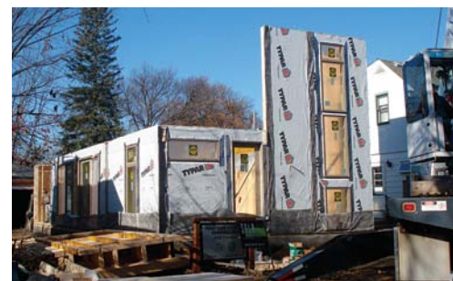
A house in a day. Wall panels arrive at the site with sheathing, windows, and housewrap installed. Insulation and drywall are added once the structure is dried in.
