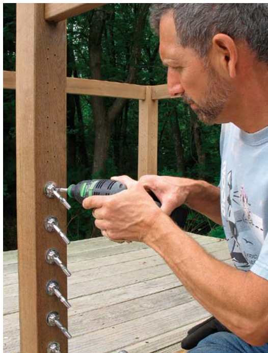
Mount all the hardware. The surface-mounted swivel fittings and tensioners shown here are mounted to the posts before pulling and cutting the cable. Because of this, you can mount all the hardware at once. Be careful not to snap or strip the stainless-steel screws by driving them too fast into hardwoods like ipé. Bored deep enough, pilot holes save headaches if they prevent even one broken screw.
