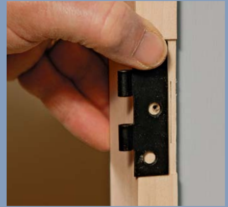
Shift one hinge. By moving the location of the hinge diagonally opposite the problem corner, it's possible to make the door land evenly on the strike. Mark the leaf location before moving it.
