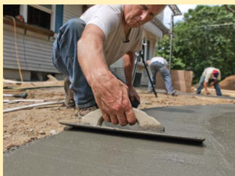
Bring up the cream. A smaller float made of magnesium, aluminum, or wood brings cement particles and fine aggregate to the surface. The resulting cream fills small voids and smooths the surface.
