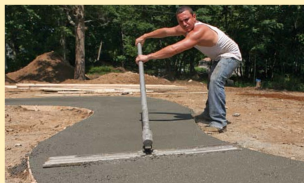
Bull float first. Take two or three passes with a magnesium bull float to level the surface and to push the aggregate into the mix. Raising the leading edge of the float will prevent it from digging into the surface. Additional handle sections provide extra reach on large pours.
