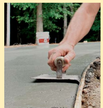
Edge the corners. After mag-floating, use an edging tool on the slab corners. Rounded edges resist weather better than sharp corners.
