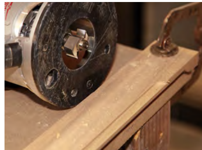
Rabbet holds the glass. On the back of the outside sash opposite the routed profile, rout a 1/8-in.-deep rabbet that will keep the 1/4-in.-thick glass centered in the sash. Once the profile and rabbet have been routed, trim the sash stock on the miter saw to final length.
