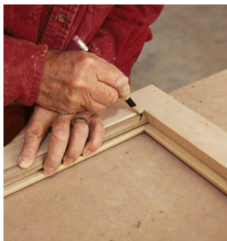
Take the guesswork out of cutting angles. To avoid confusion when cutting the glass stop, set the stop in place in the sash frame and mark the angle of the cut.
