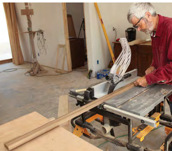
Mill the glass stops. Using the same router bit as you used on the outside sash, with the cutting depth set so that the profile has only one shoulder, rout the profile on the edge of 1/2-in.-thick stock. Then rip the stock to 1/2 in. square to create the stop.
