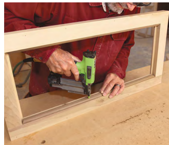
Temporary home for the stops. The glass stop is not installed for good until the painter is finished, so tack each length of stop in place with a headless pin. When the glass is in place and the stop is installed, the stop will leave a 1/8-in. shoulder to match the profile on the other side.
