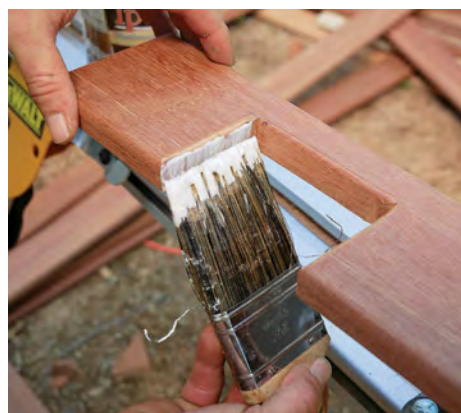
Seal end grain. Apply sealant (we used DeckWise lpe Seal end-grain sealer) to the end grain of the post notches and the ends of the treads to minimize water absorption.
