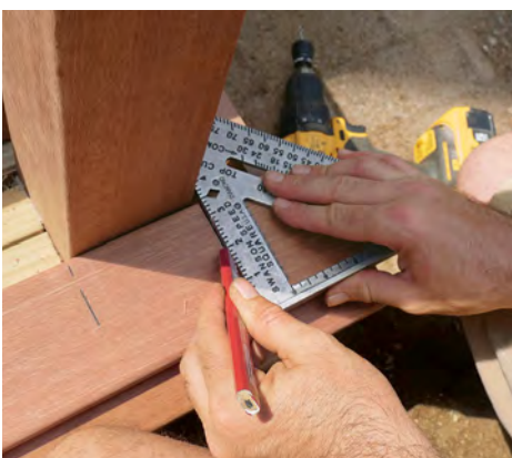
Notch for posts. Use a speed square to transfer post locations to the tread boards of the bottom step. Cut the notch with a jigsaw and round over the cuts.
