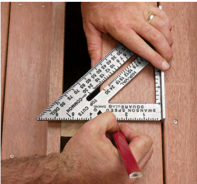
Create even gaps. When installing the cut and routed tread boards, a speed square is used for gapping and marking screw placement.
