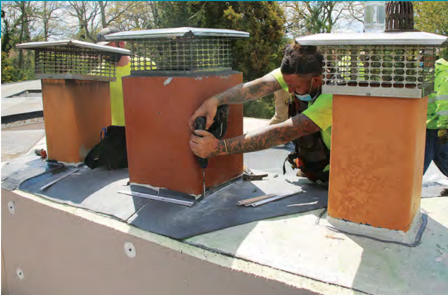
Fix a leaky chimney. The chimney can't be seen from the ground, so it made sense to insulate it and cover it with EPDM so it could be more reliably flashed and in order to reduce thermal bridging. The insulation is held to the masonry with concrete screws. Drive anchors hold the termination bars.
