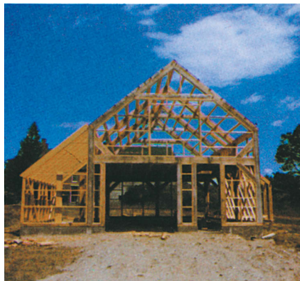
A modern saltbox under construction in upper New York state. Framing is basically traditional, but the common partition between Cape and shed has been replaced by posts and beams to open up the interior. Photo: Patsy Hennin
