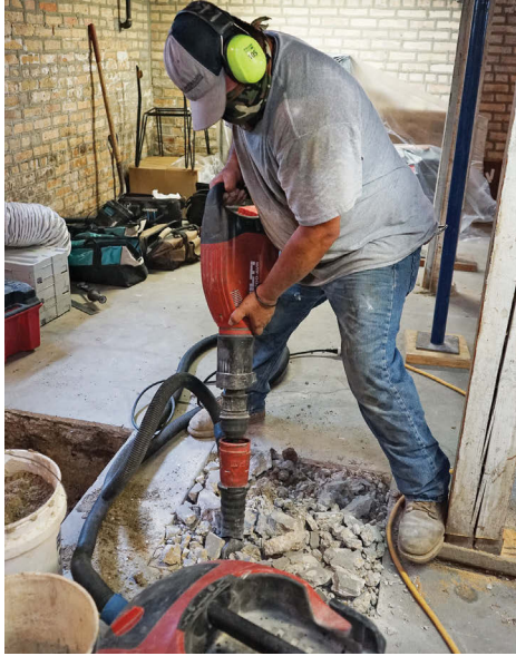
Source collection. The crew uses saws and breakers equipped with dust-collection systems that handle most of the fine dust from cutting concrete.
