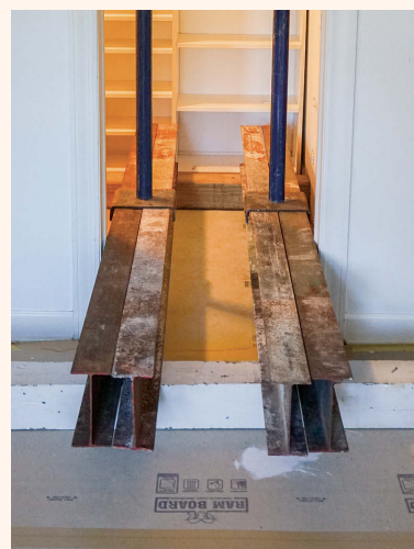
Tight quarters. When there isn't enough room to spread the load in a tight space, crisscrossed layers extending to larger spaces can be used to support the loads.
