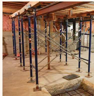
Bottom up. Shoring installation starts in the basement and continues upward to support the structure around the failed member. After standing up the shores and before raising their screwheads to the floor or ceiling above, we place beams on top of them to spread the weight among multiple joists.
