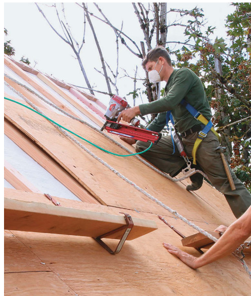
Sheathing completes the channels. Roof sheathing is fastened as usual, creating a deck where roofers won't encounter any uncommon details.
