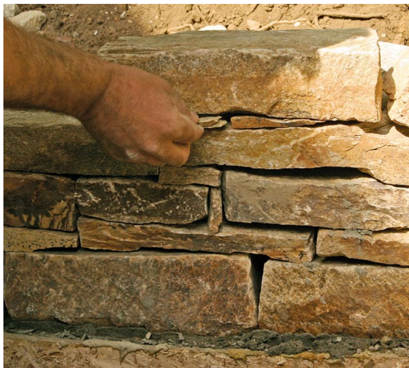
Gaps get scraps. To help create a true dry-stack look, we use the chipped-off chunks and slivers from our rock hammering to fill the spaces between stones. Ideally, these small stones will slide in deep enough to be held in place by the mortar. If not, add a bit of mortar before inserting.
