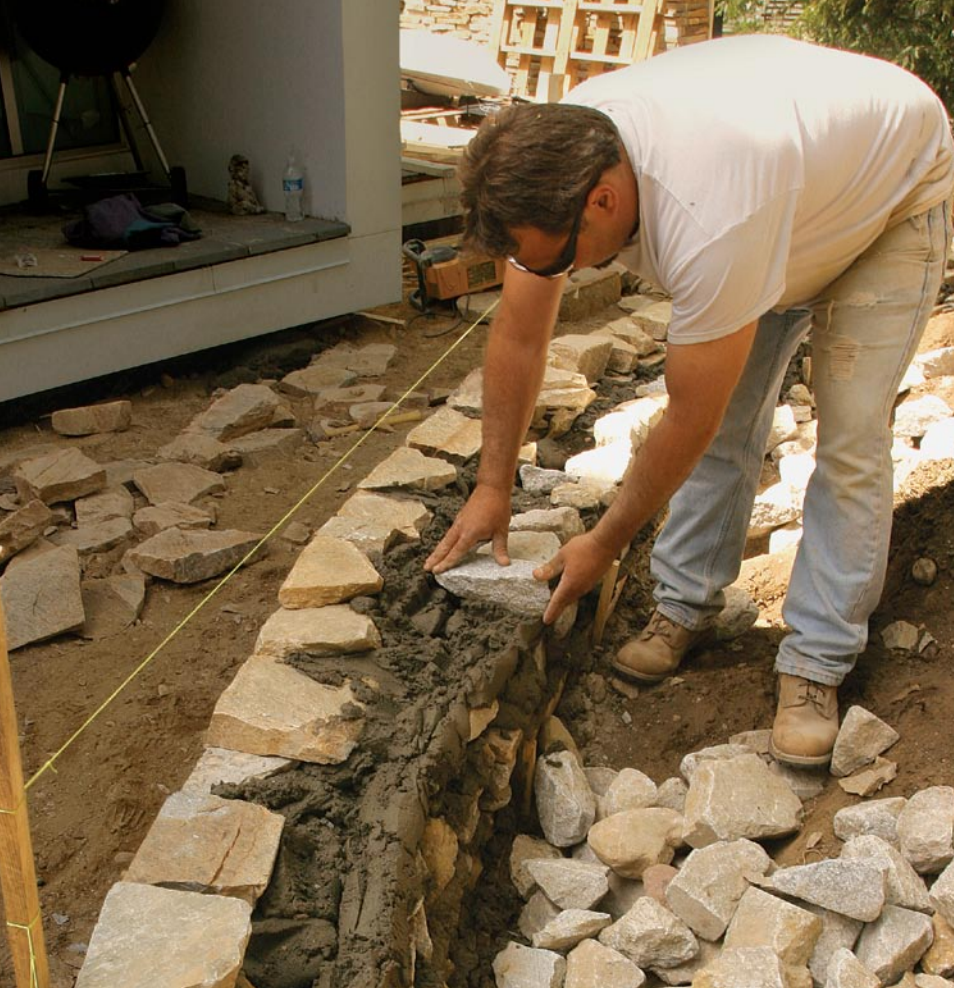
Build up the back side. After setting a few courses of stone on the face of the wall, I build up the back side with less expensive blasted ledge stone set in plenty of mortar.
