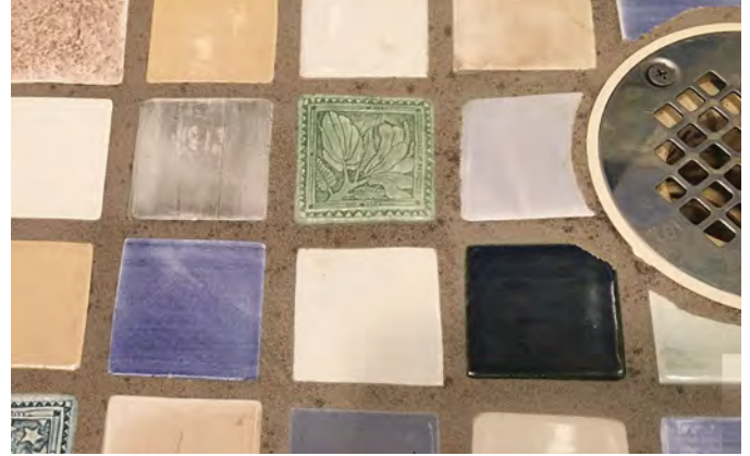
Nine-year-old polyurethane grout showing black spots from regular use.
