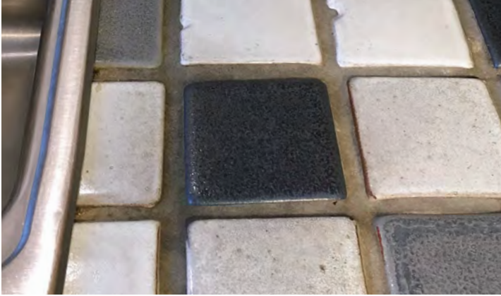
Seventeen-year-old epoxy grout showing food and water stains.
