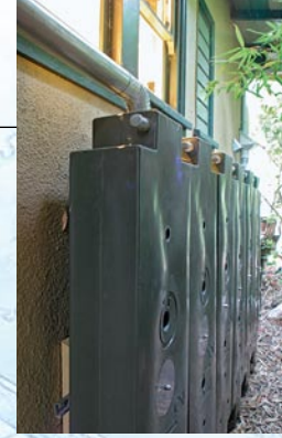
On the north wall, modular tanks linked together store rainwater piped in by way of the roof's gutters and downspouts.
