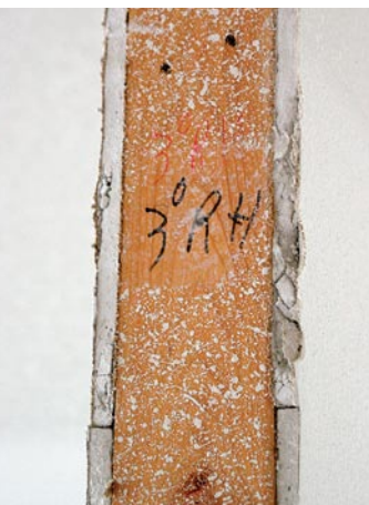
Size and swing. Write the door size and swing on the hinge-side trimmer stud of each rough opening before the drywall is installed.
