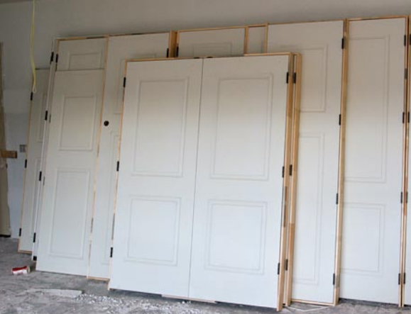
Hinges face away from the wall. On concrete floors, a vapor barrier protects doors from moisture. Here, the barrier is not in place yet.
