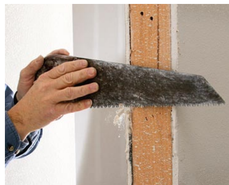
Clear all potential obstructions. Trim back the drywall on both edges of each trimmer stud using a rough-cutting handsaw.
