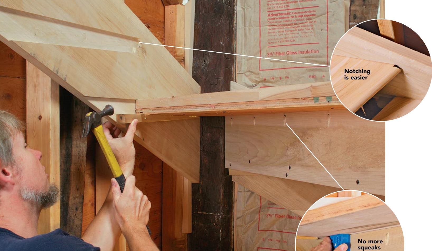
New ways combined with the old. Each winder, with subtread attached, was slid into the mortises and locked in place with a wedge slathered generously with glue. At the front of the winders (top inset), the nosing was notched rather than housed to simplify construction. Underneath (bottom inset), pocket screws drew the treads tight to the risers.
