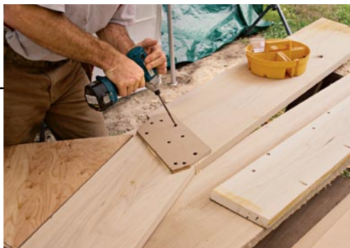
To accommodate the shallower pitch of the winding treads, the upper wall stringer was made in two pieces. The joint was reinforced with biscuits and a plywood gusset on the back side, and was screwed to the house framing at installation.
