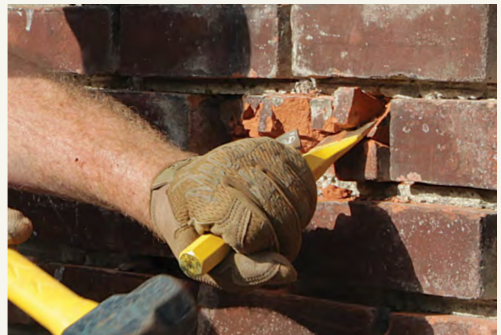
Chisel 'em out. Use a hammer and wide masonry chisel to slice out the pieces of broken brick. Removing the top half of the broken-up brick first provides room and relief to easily remove the bottom half without pressuring and possibly breaking the surrounding brick.
