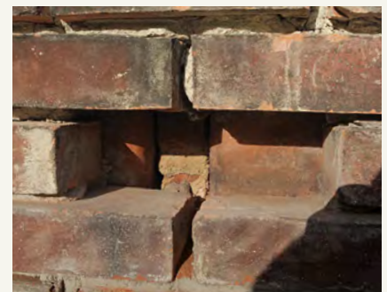
Reason for care. Many chimneys are only one-wythe thick, with the masonry flue right behind it. Be extremely careful not to damage flues, especially if they're in active use.
