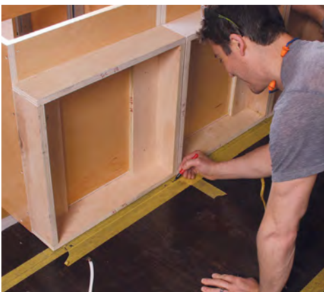
MARK FOR BLOCKING With the island cabinets screwed together and on their backs, we mark the locations of the cabinet sides for floor-mounted blocking.
