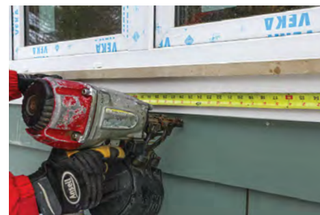
Nailing cutouts. Where siding is cut to fit under windows, face-nail 8 in. o.c. using the same 8d nails used for blind-nailing. Flush nails can be painted; overdriven nails need sealant.
