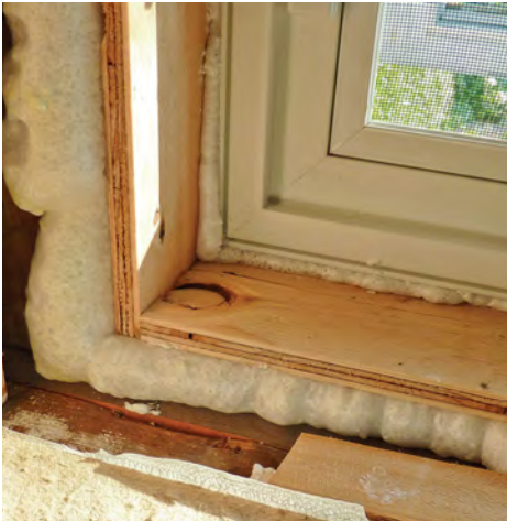
Foam the gap. Sprayed into the spaces between the box and the framing and between the window and the box, expanding foam both air-seals and helps to support the assembly.
