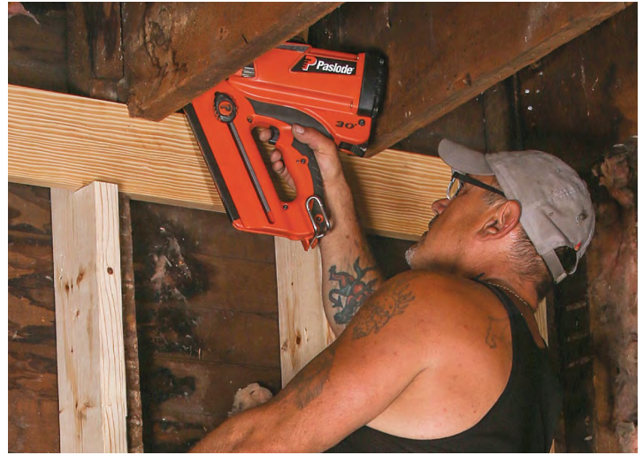
Attach the joists. When the floor is settled onto the new lower ribbon board, nail the joists to the sides of the studs.
