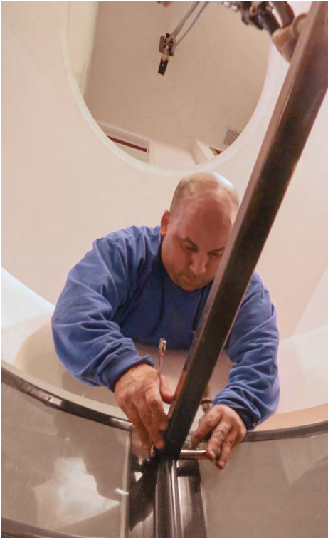
Preparing for lift. The hoist chain is attached to a temporary steel rod, which is fastened to a ring with metal pins.
