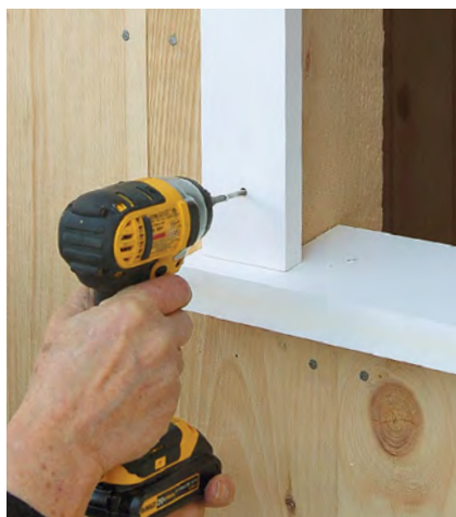
Trim the barn-sash opening with PVC. Install the angled sill first, followed by the casing legs. The casing overlaps the opening by \frac{3}{4} in.
