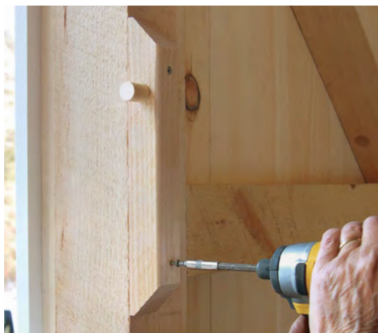
Install the barn-sash keepers. Screw foot-long pieces of 2-in.-thick pine, with \frac{3}{4} -in. dowels installed in them, to the inside of the posts. This provides a stop for the window sash when open.
