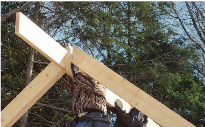
Raise the ridge. Like the plate beams, the 2x10 ridge is 20 ft. 4 in. long. After marking the rafter layout to match the plates, push the ridge up between the rafters, and secure each rafter to the ridge with two 6-in. screws. Install the remaining rafters.
