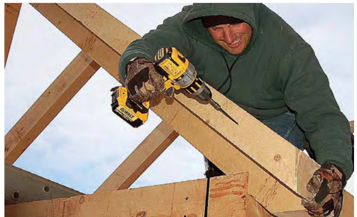
Add the four 4x6 fly rafters. The fly rafters are the same length as the main rafters, but they have no bird's mouths. Hold them against the gable-end roof rafters with their top edges flush, and fasten them with 10-in. screws about 16 in. apart.
