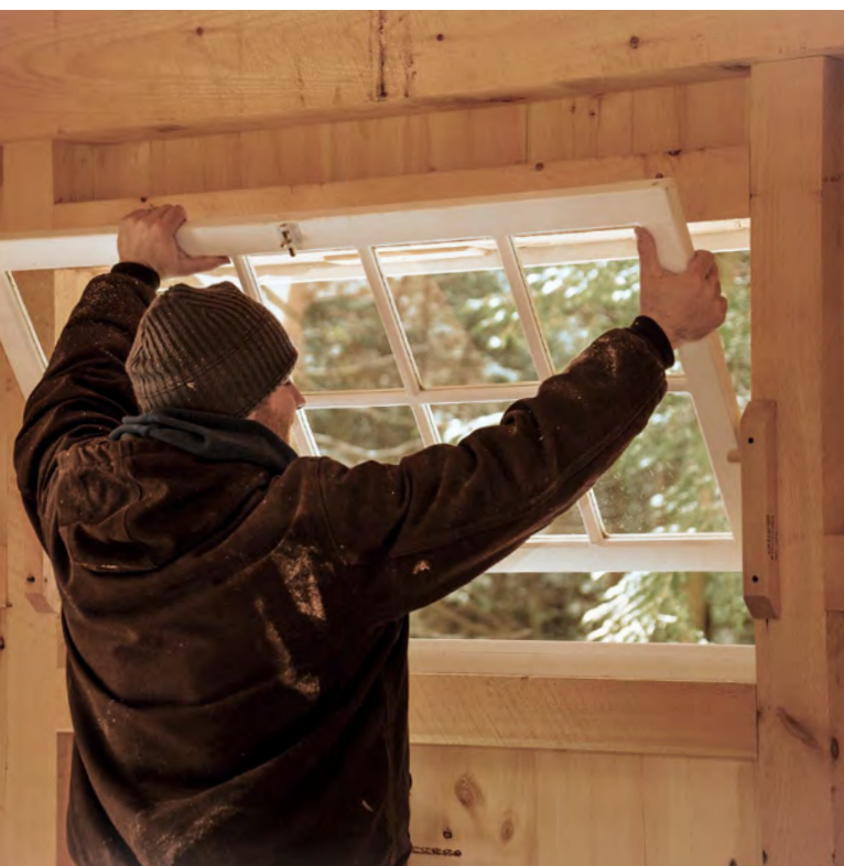
Set the sash. The barn sashes simply slip into place. A small barrel bolt at the top of each sash keeps it closed.
