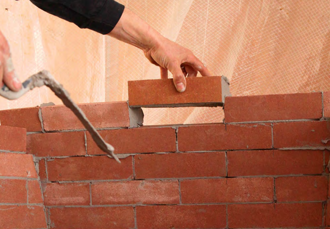
Head lock. Work from the outside in as the curve gets steeper; the mortar in the head joints—those on the ends of the bricks—helps keep individual bricks from sliding off. The exposed bed joints in the curve should have the same thickness as the bed joints in the courses that were laid level.
