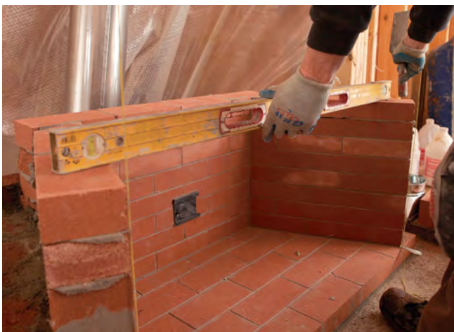
Level across. Lay a long level across the sidewalls for each course, and tap down bricks as necessary to keep their heights even.
