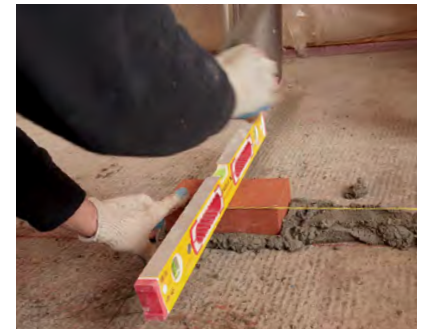
Work from the center out. Lay the end of the first brick for the hearth on the centerline, and level it both along its length and width.
