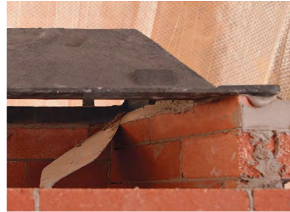
Bevel the edge. From below, use a small trowel to neatly bevel the mortar joint between the walls and the damper.
