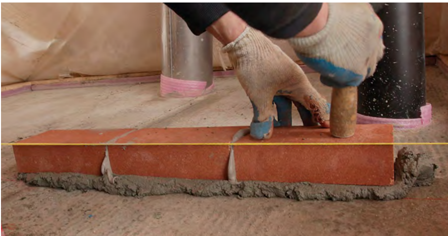
Line and stick. Use a stringline as a guide to keep the bricks in line and in plane as they're tapped down to the proper elevation.
