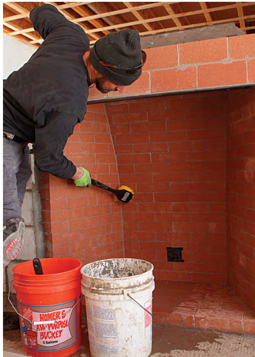
Clean it up. Once the joints are set, sponge off the bulk of the excess mortar, then use a brush and a diluted solution of acid-based cleaner and water to scrub the walls, and immediately rinse with clean water.
