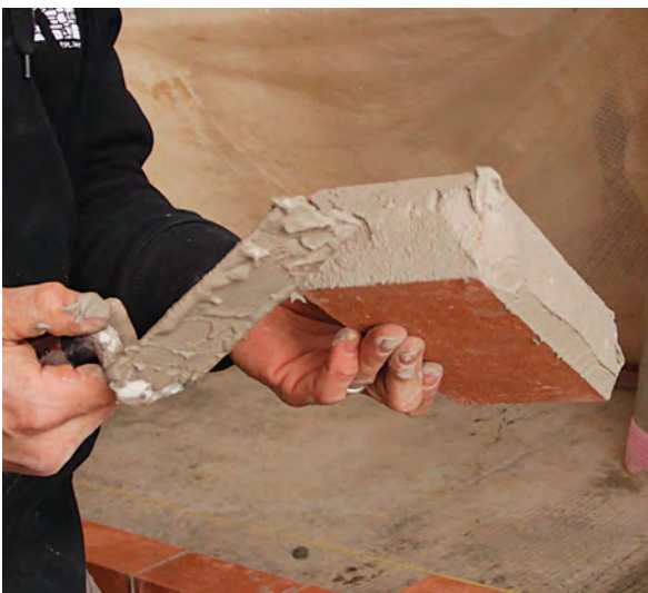
Don't get sloppy. Trowel on enough mortar to fill the joints—roughly \frac{1}{8} -in. thick—and bevel the edges to avoid excess squeeze-out.
