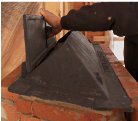
Allow for expansion. Leave a 1/4-in. gap between the damper and the brick atop the lintel.
