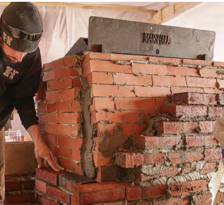
Backer up. Use less expensive backer bricks and Type-S mortar behind the firebrick lining of the firebox.
