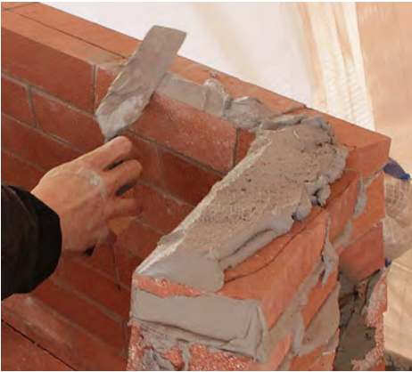
Ready to cap. Dry-fit the damper, trace its perimeter, and then remove it and apply refractory mortar inside the line.
