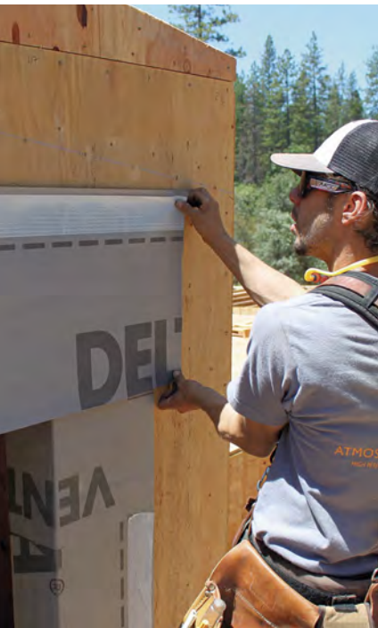
Shingle-flash the opening. With the head flashing in place, Delta flashing tape on the sill and corners ensures the integrity of the air and water barrier.
