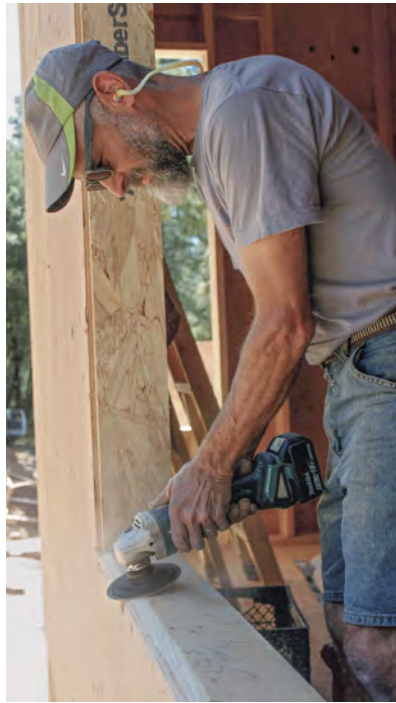
Bevel the sill. Dave takes a grinder to the sill to provide positive drainage to the outside.
