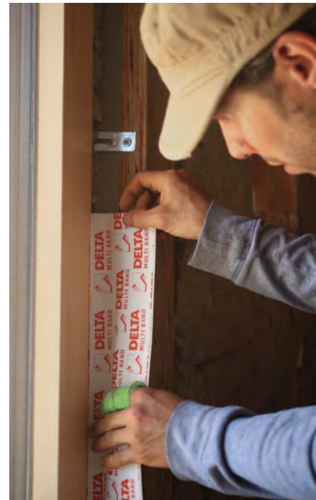
Tape the edges. On the outside, the window head and jambs are sealed to the WRB with tape. After filling the cavity with insulation, the interior is taped on all four sides.
