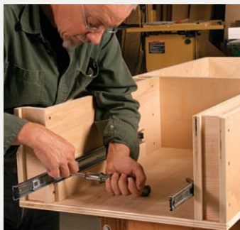
Install full-extension drawer slides. Place the slides atop a spacer block during installation to ensure correct alignment.
