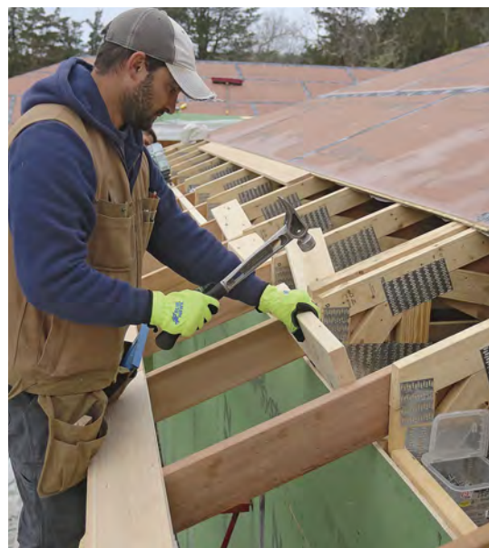
Blocking for insulation. In each truss bay, 2x6 blocking provides a backing for the closed-cell spray-foam insulation.
