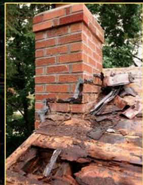
1 A little bad flashing can cause a lot of damage. This roofer cuts the patch stock in place after nailing one end of the board. His sawblade is set to the depth of the patch stock.
