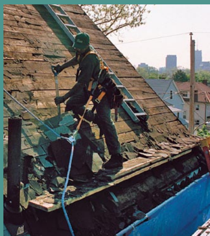
A safe setup makes the job go more quickly. Tied off to the ridge, this roofer has the extra peace of mind that a misstep won't be fatal. The roof ladder provides safe footing while tearing off from top to bottom.
