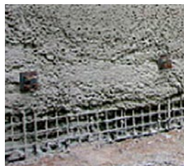
Tightened nuts embed an 8-in. steel plate into freshly sprayed concrete. More concrete is sprayed on to cover the hardware.
