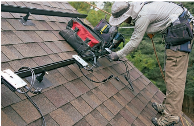
Optimization stage. A power optimizer is mounted at each module location, each one locked to the rails with T-bolts.
