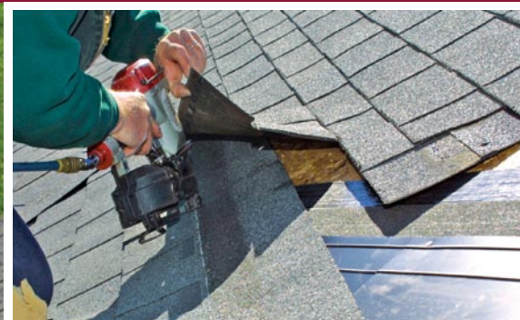
Keep nails out of the valley. Lay shingles over the valley flashing to be cut later. The existing shingles provide a layout guide.
