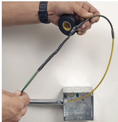
Stagger the wires. After running the fish tape between pull points, prepare the wires by staggering their ends. One should be about 3 in. longer than the rest. Feed this long wire through the fish tape's eyelet, and bend it back until it's just shy of touching the tip of the next-longest wire.
