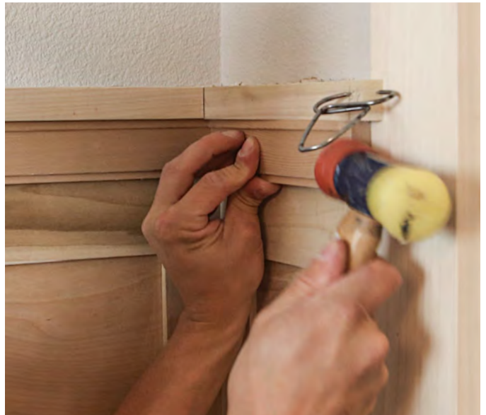
Finishing touches. Wrap up the installation with a panel molding under the cap. Return its ends, tap it into place, and fasten. The rest of the job is left for the painters.
