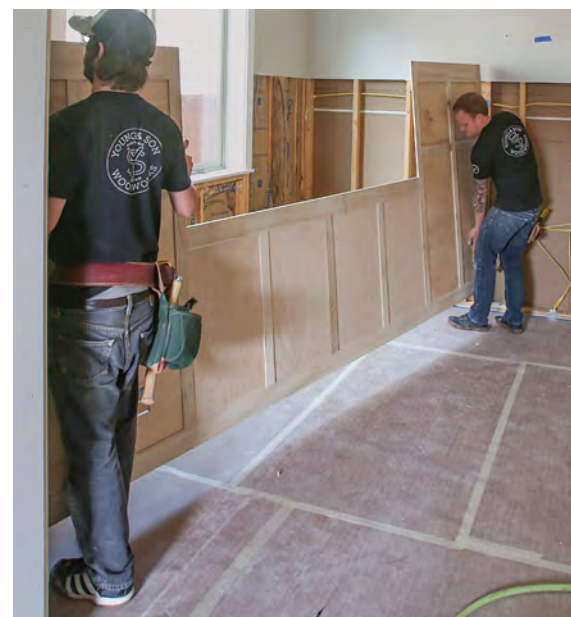
Moment of truth. With the fitting done, walk the panels into place, where they will be positioned for fastening.
