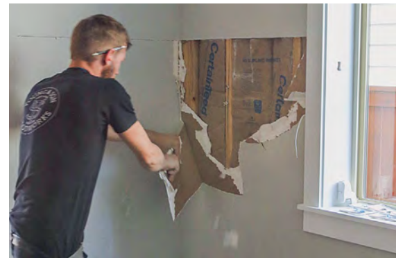
Clear the way. Remove all the drywall in the area to be wainscoted. Once the studs are fully exposed, take out the drywall screws.
