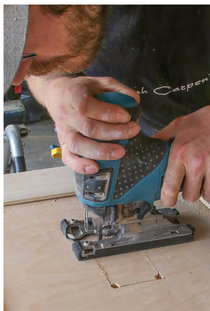
Connect the dots. Cutouts for electrical boxes are done on site by drilling holes at each corner and cutting between them with a jigsaw.
