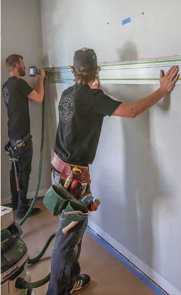
Clean, straight cut. Use a helper to hold a straightedge to a laser-level line, and cut the drywall using an oscillating multitool. Hold a vacuum below the multitool to catch dust.
