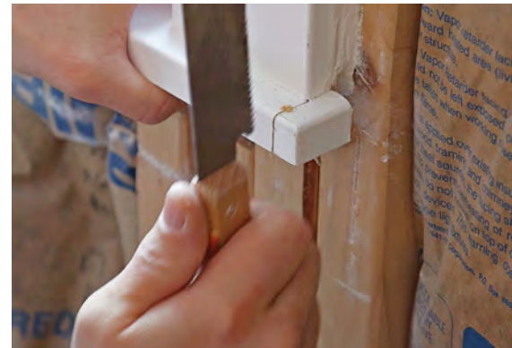
Remove hang-ups. Cut window stools flush with the casing to allow the panels to be placed. These offcuts can be glued back in place after installing the wainscot panels.
