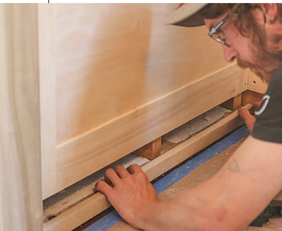
Pad the base. Nail scraps of frame material in place to pad out the bottom of the wall behind the base molding.
