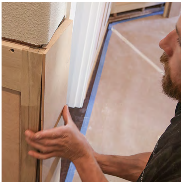
Small walls get solid panels. Rabbet the panels' backs to keep each panel's edge flush with the face of the abutting panel.
