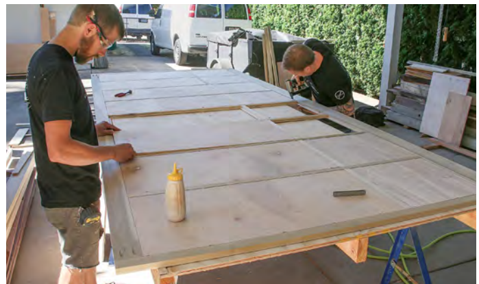
Build it backside up. Cut intermediate rails to length and fit them between the stiles. Attach them with glue and corrugated fasteners. Glue and staple the plywood panels into the rabbets.
