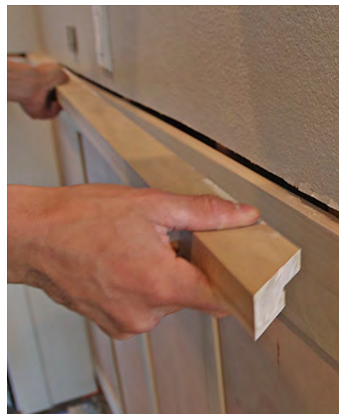
Clean cap. The cap's rabbet ensures it sits at a consistent depth. Miter the ends and nail the cap to the top rail.
