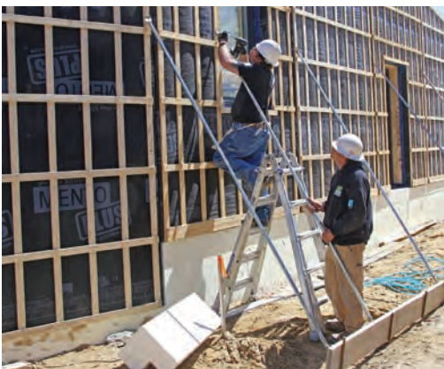
Plumbing and bracing. Adjustable steel bracing from Qualcraft makes it possible to plumb panels and keep them safely upright. 2x10 boards at grade level allow for more-flexible mounting locations, and the steel form pins that support the 2x10s easily penetrate rocky soil.
