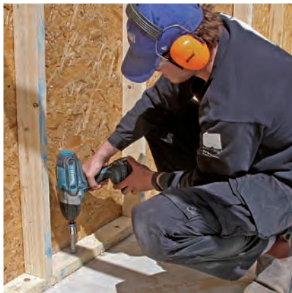
Anchors act as hold-downs. Simpson Titen HD anchors spaced every 2 ft. hold the wall panels to the slab foundation. The 1/2-in. holes are made with a rotary hammer and the anchor is tightened with a 1/2-in. impact wrench.
