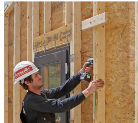
Structural screws join panels. GRK structural screws join the panels to each other and to the beams and posts. Wood cleats screwed to one of the studs where the panels join help correct any misalignment at panel edges.
