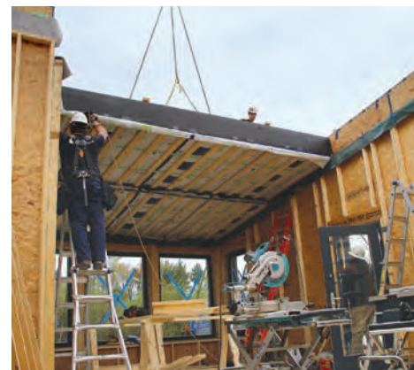
Roof panels install like floor panels. Roof sections are constructed and fastened similarly to floor sections, except they contain a cellulose insulation layer like the wall panels. A double bead of Contega sealant stops air leaks at top plates.
