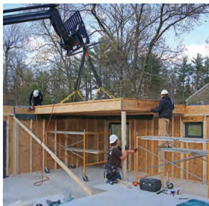
Panels make framing different. Unlike typical platform framing where beams supporting the floor system are installed ahead of the joists, here the floor panels are temporarily supported until beams can be screwed to the panels.
