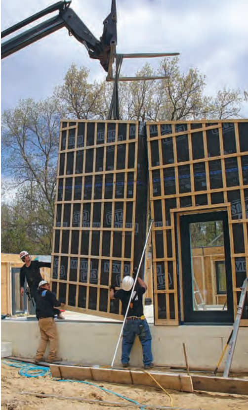
Machine muscle. Each panel weighs between 600 lb. and 1200 lb. and must be handled with machinery. Double beads of Contega sealant on the foundation and between the wall and roof sections stop air leaks. Panel joints are also taped for air- and weathertightness.
