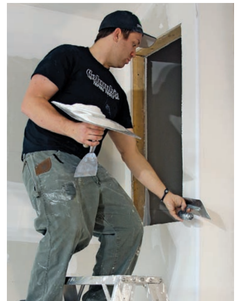
Handwork is still required. Automatic tools can finish a large part of the job, but you still need to know how to use hand tools for corner beads, repairs, and tight spots, like this AV equipment built-in.
