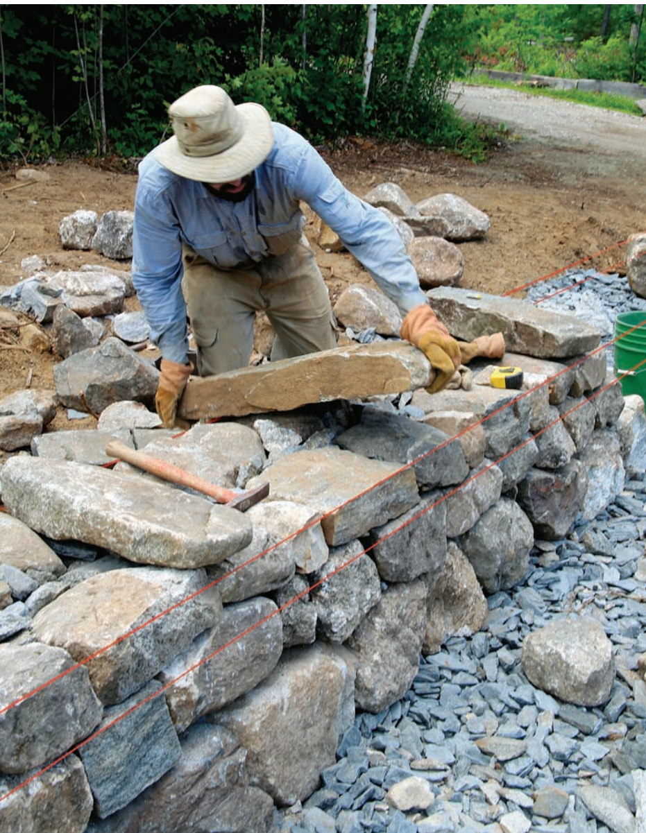
Tie the sides together. It's typical to let through-stones extend 1½ in. past the wall face to allow for flexibility in their length and for the wall to settle without slipping off them.
