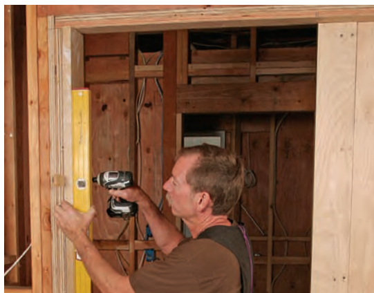
Fasten the strike jamb. Using opposing shims, plumb the strike-side jamb, and fasten it every 8 in. with pairs of trim-head screws. A 6-ft. level ensures that the jamb is straight throughout its length so that it will make full contact with the edge of the door.
