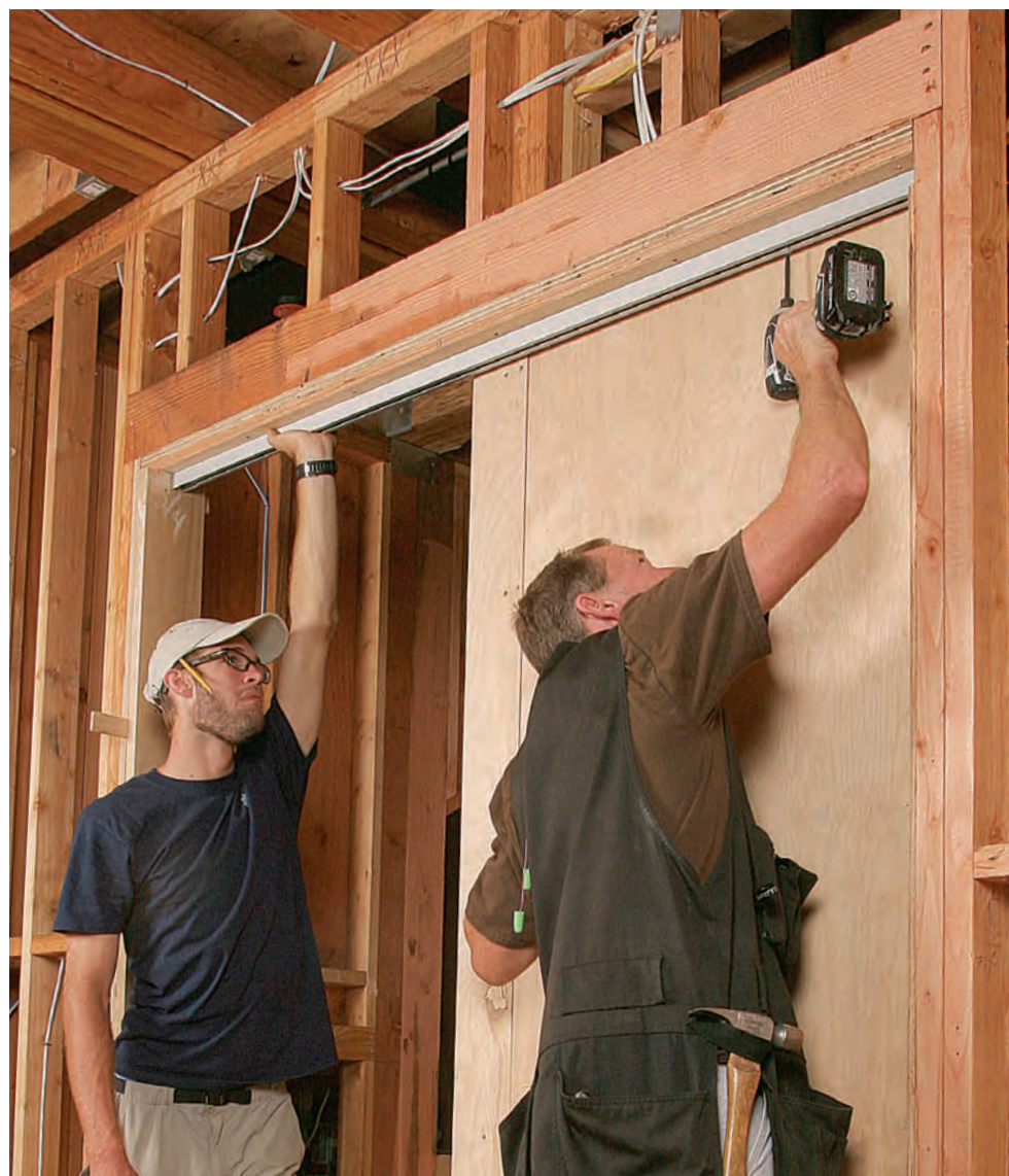
Install the track. Fasten the track to two layers of \frac{3}{4} -in. plywood attached to the bottom of the structural header. The plywood provides a straight, twist-resistant surface and bridges the gap that's in the center of a two-ply header, which is where the track-mounting screws go.
