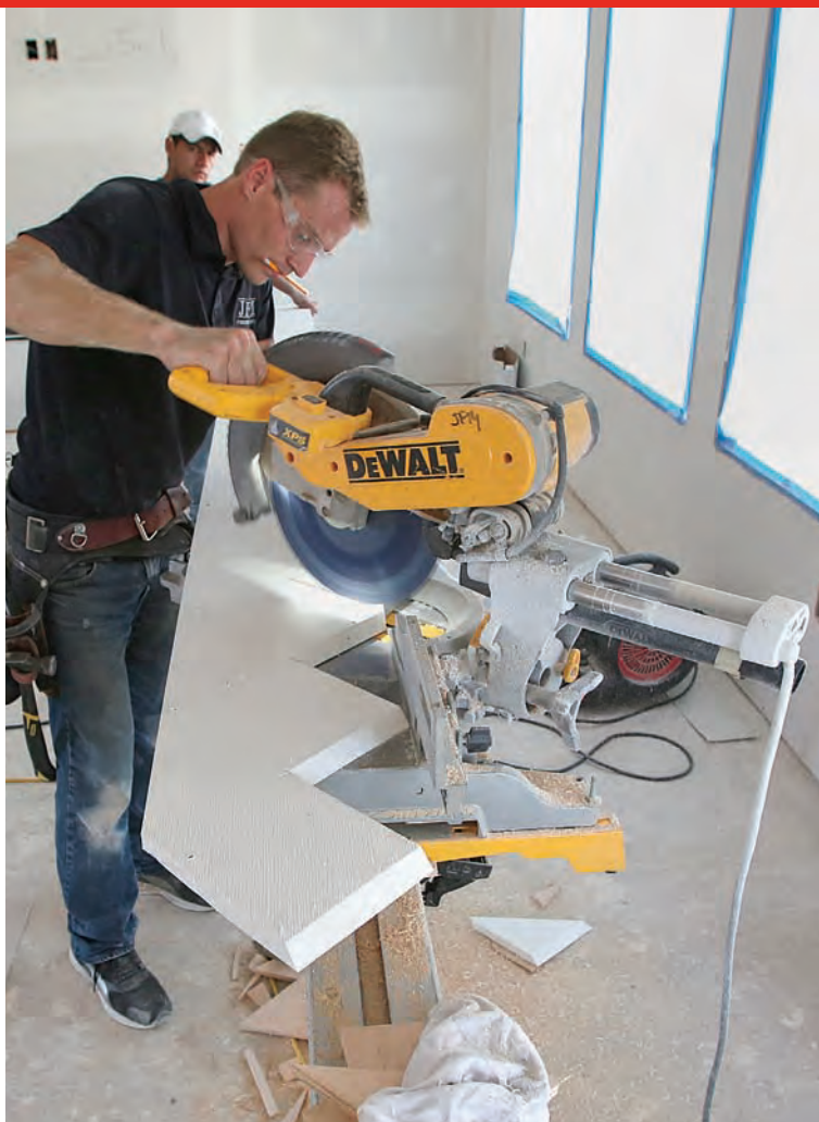
Easy notching. Laid out flat, the skirtboard can be notched using a sliding miter saw. The tread cuts are straight 90° chops, but the saw is beveled to make the riser cuts so that these edges can be mated tightly to the finished riser stock that comes later.
