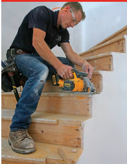
Prep the rough stairs. Radius-edged rough treads are cut flush to the rough risers to create an accurate reference point for measurements and to clear the way for the false tread caps that come later.
