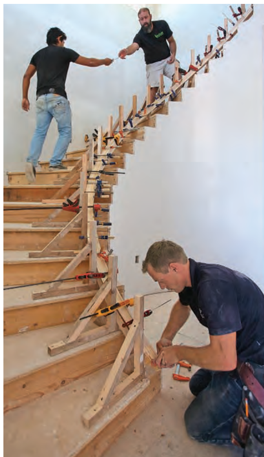
Aim for a fair curve. After its laminations are coated with wood glue, the poplar handrail is sandwiched together, held with a few bands of shrink wrap, and pressed into place against the form. When the rail is properly positioned, it should be tight to the face of each bracket, set down against the angled stops on each bracket that match the slope of the stairs, and twisted so that the bottom face is flat to the top of the treads. Holding the rail tight to all these critical areas requires a lot of clamps, so have plenty on hand.
