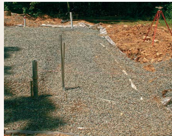
Graveled and ready for foam. Strings between batter boards define the foundation perimeter. Conduit for electrical and phone lines is in the front, while stubs for plumbing stick up in the back. Perimeter drains are visible along the right.
