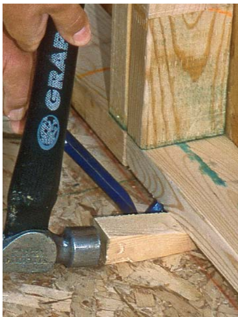
Shim the bottom plate. To correct imperfections in the floor framing, drive a wedge under the bottom plate. When the top plates are level, nail the wall sections together, and remove the shim.
