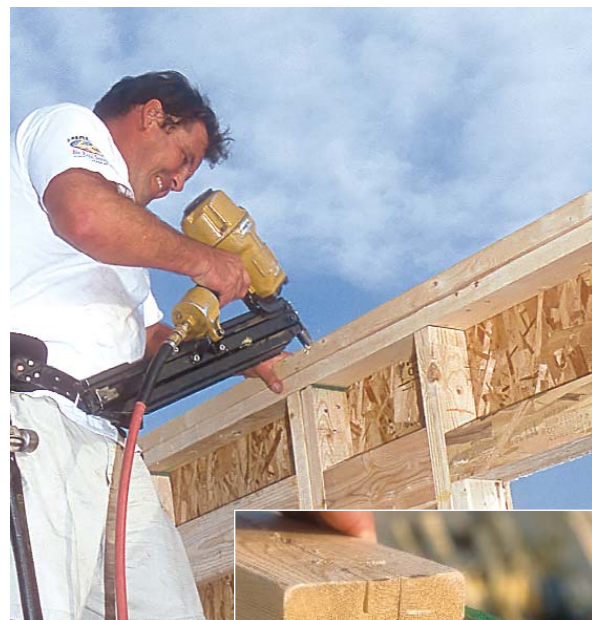
Add the double plate over wall intersections. Make sure to bridge the intersection of two wall panels with a double top plate. The top plates are marked for intersecting walls (inset photo).
