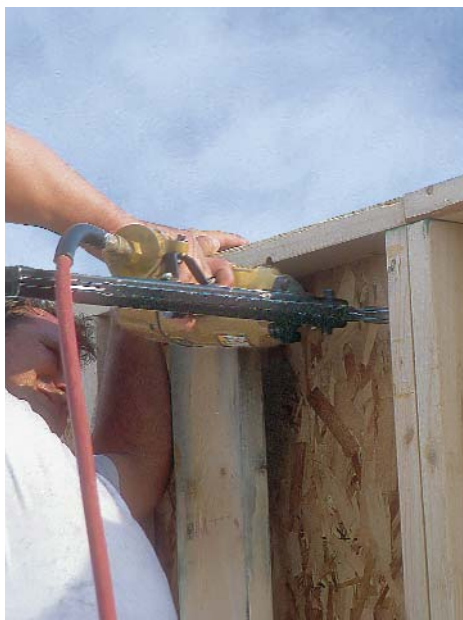
Nail the end studs together to join wall sections. When the top plates in adjoining panels are level and flush, nail the end studs together with 16d nails.
