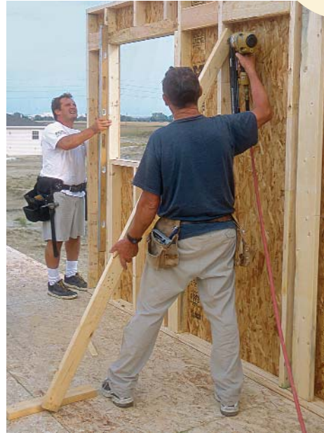
Plumb and brace each wall section. As you set the wall sections, check them for plumb, and temporarily brace them with a 2x4 every 8 ft. to 12 ft.
