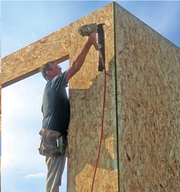
Nail off the intersections from outside. The wall sheathing extends over intersections and corners to create a structural splice. Nail the sections together from the outside.
