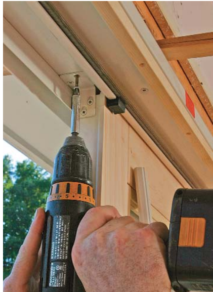
Gravity and metal brackets hold the fixed panel in place. The shims above the jamb are temporary. They allow the author to snug up the bracket. The top jamb shouldn't be shimmed permanently to allow the house to move without disturbing the glass doors.
