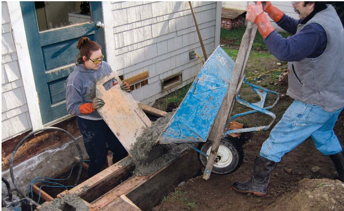
Buggy-pouring is easier with a helper. A strategically placed helper with a splash board gets the mud inside the forms with fewer spills. If you can't persuade your daughter to help you, brace and nail the splash board in place.
