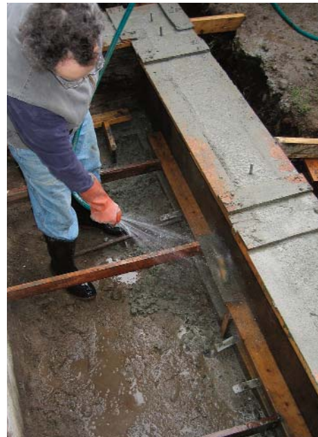
Clean the forms while the concrete is wet. Stripping goes more quickly if you don't have to chip away hardened concrete to find the nails. Another way to make stripping easy is to use two short boards rather than one long board when building the forms. This reduces the effect of pressure exerted by concrete on the inside-corner joints.
