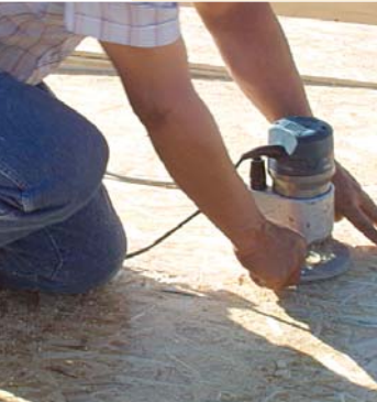
A router removes exterior sheathing at window and door openings. To follow the framing around the opening, you need a plunge-cutting straight bit with a bearing beneath the cutter.
