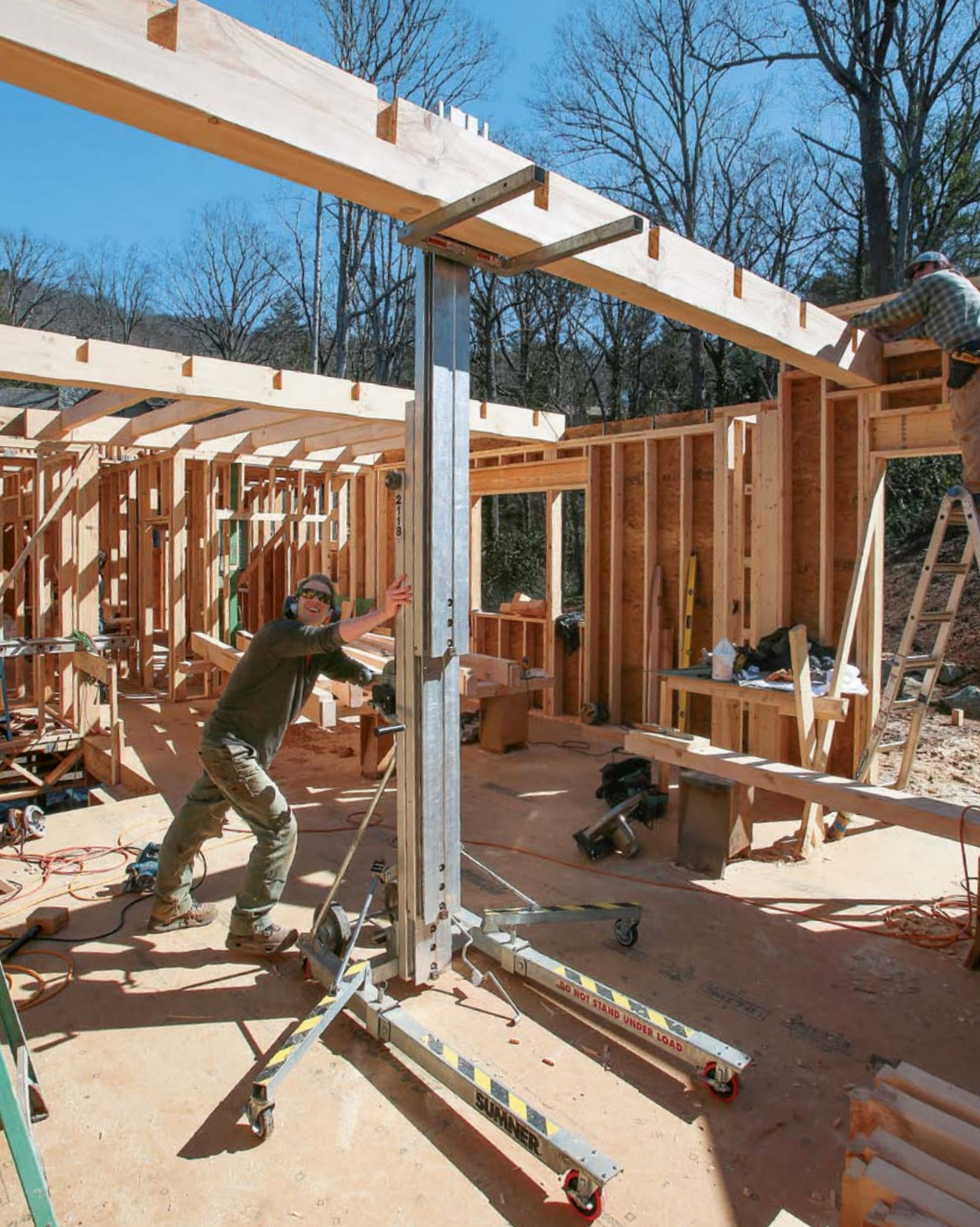
Easy lifting. A wheeled material lift, available from rental yards for about $60 a day, makes quick work of lifting the beams and joists into position.
