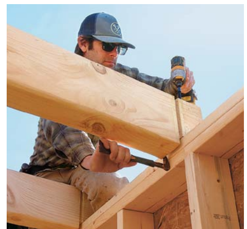
Screws for the plates. With the drywall groove aligned to the interior face of the stud wall, a single structural screw (TimberLoks were used here) driven through the top of its end secures the joist to the top plate below. Because the lumber is wet, no pilot hole is needed.
