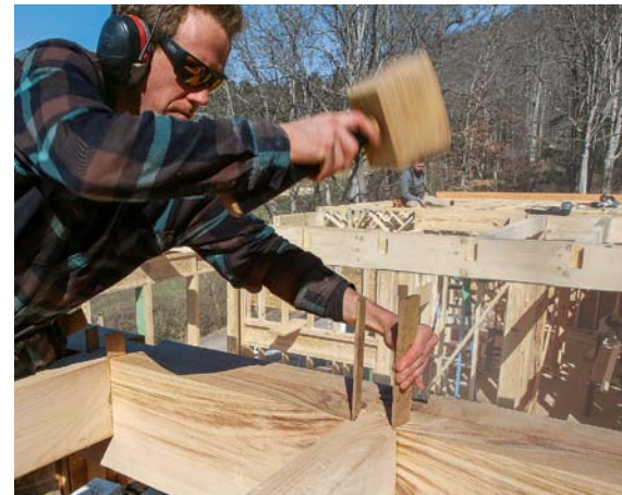
Shims for the tenons. Untapered oak shims draw the shoulders of the joists tight against the beam face, locking the joists into place.
